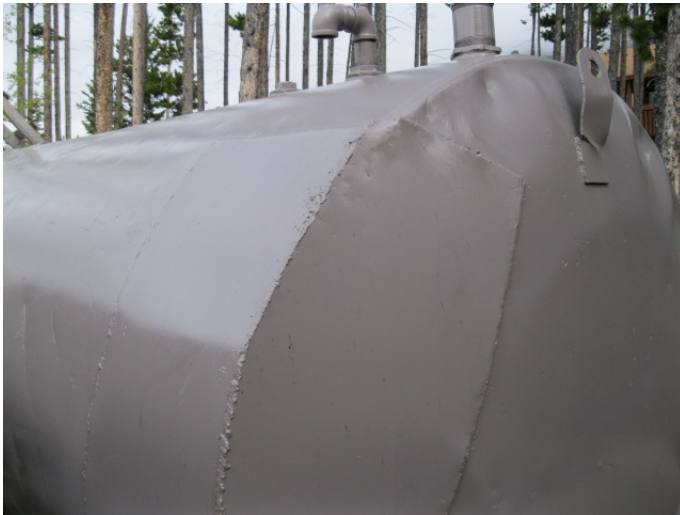
UST installed aboveground
